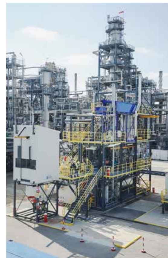
ReOil plant on OMV's Schwechat site
